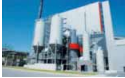
In 2010, Stora Enso commissioned a new 140 million Euro multifuel boiler at its Langerbrugge pulp and paper mill in Belgium. With an annual input capacity of 250000 – 300000 ton biomass and Refuse Derived Fuel, it generates 125MWh of power. Photo: Stora Enso
