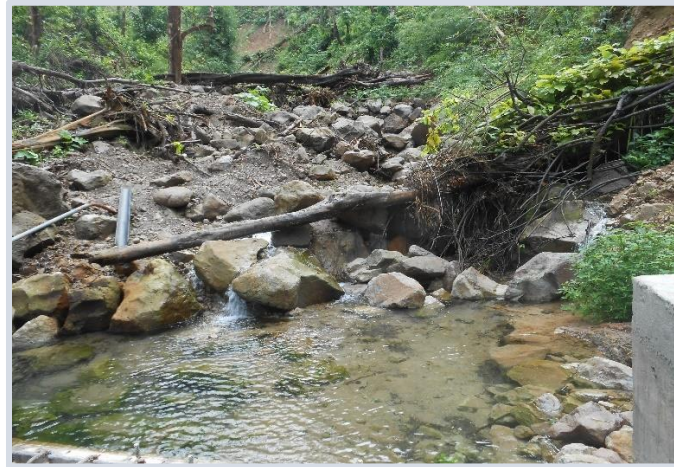
Figure 3 River damming by Forest debris, 2017 (Source: Dominica Forestry Division)
